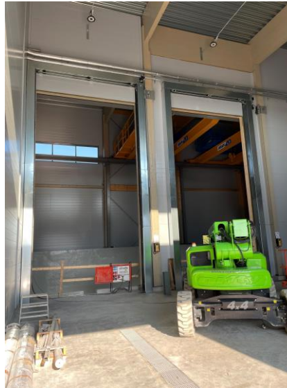
Rullportar i mottagningshall
